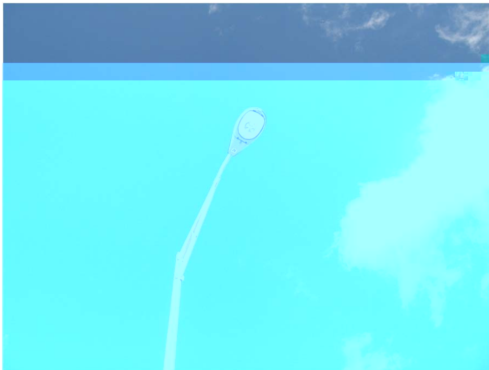
Example of Cobra Head LED Retrofit Unit (Holly Drive and West Entrance to CPT)
